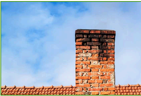
Black soot stains were noted on the exterior of the chimney, suggesting improper or problematic draft and merits further evaluation.
