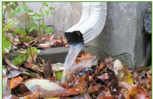
Install extension pipes, elbows and splash blocks where needed to divert the water away from the building where needed.
