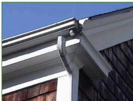
Reconnect and rivet the joints together where needed for a more secure connection.
