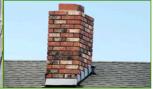
A flat chimney top (a.k.a. chimney crown) will not provide adequate rain water drainage, this condition will very likely cause cracks, damage and leaks over time. Correction is advised, the chimney crown should be sloped in a manner that would shed rain water, snow and minimize ice accumulation.
