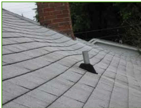
Portions of the roof appeared to be sagging, further evaluation is recommended to determine cause and repair prior to closing.
