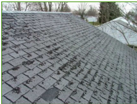
Granular layer was noted to be deteriorated, indicative of an older roof. Replacement is advised.
