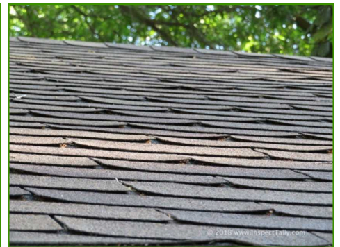
Some shingles were noted to be cupping/curling, this condition will increase your chances of problems or roof leaks in the near future. Repair/replace where needed.
