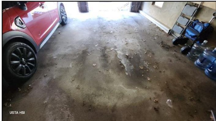
Oil staining was observed on the garage...
