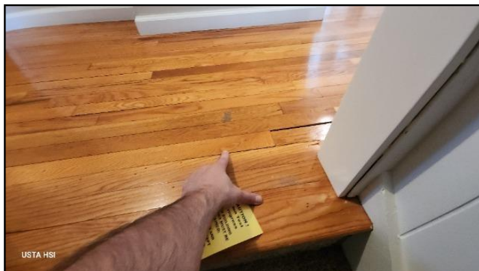
Loose floor boards were observed.
