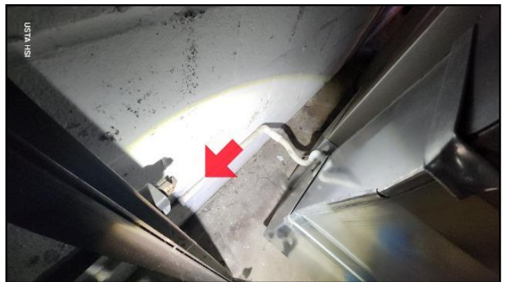
Improper discharge point observed for the...
