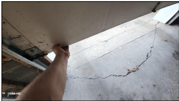
The garage door failed to auto-reverse...
