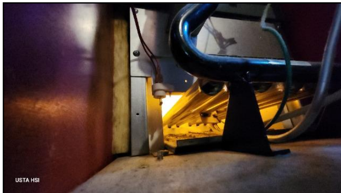
An orange flame was observed at the boiler...
