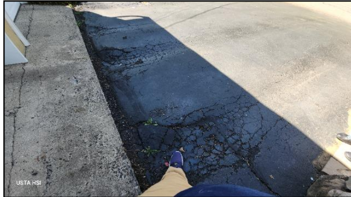
Driveway heaving observed.
