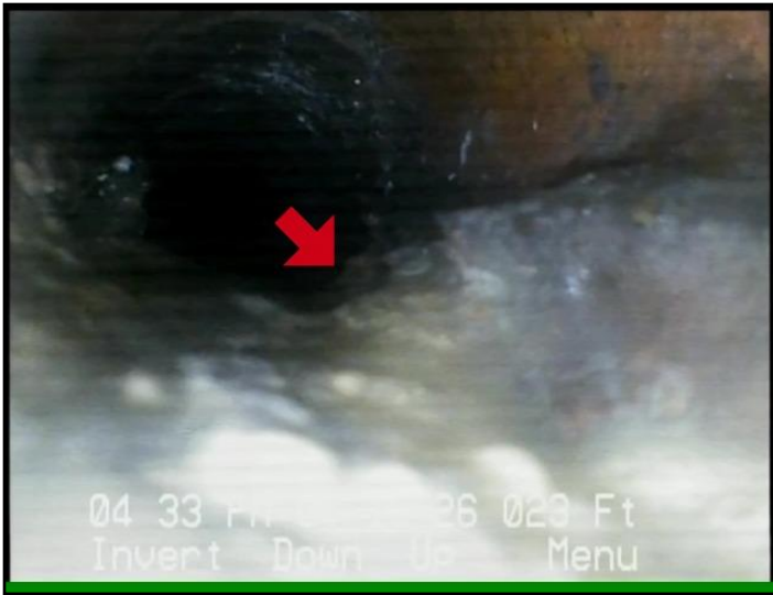
Grease buildup observed along the bed of th...
