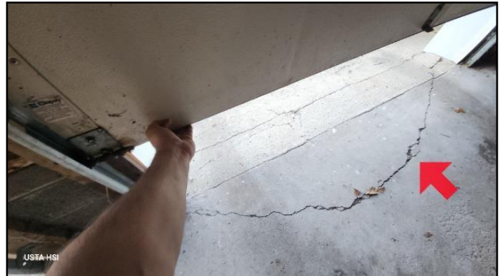
Cracking and deterioration were observed in...
