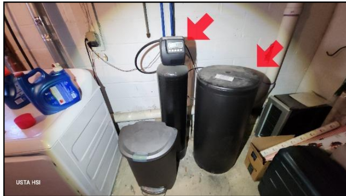
Brine tank / Water softener
