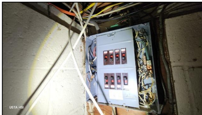
A Zinsco electrical panel or subpanel was...
