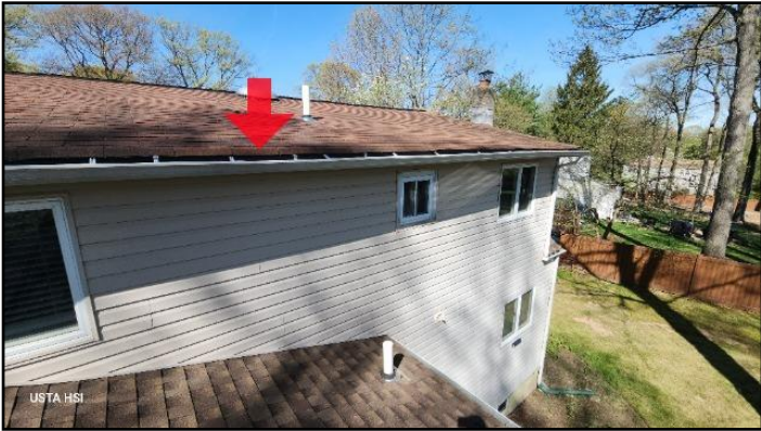
Gutters with improper slope or ponding wate...
