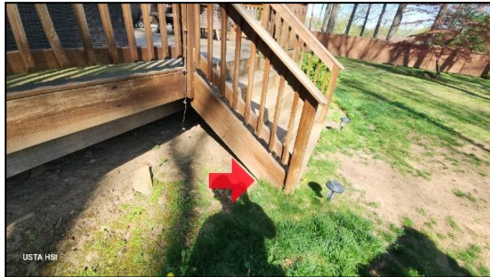
Wood-to-soil contact damage at stringers or...
