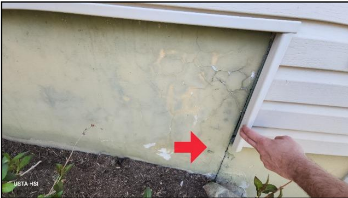
Minor cracks were observed on the exterior...
