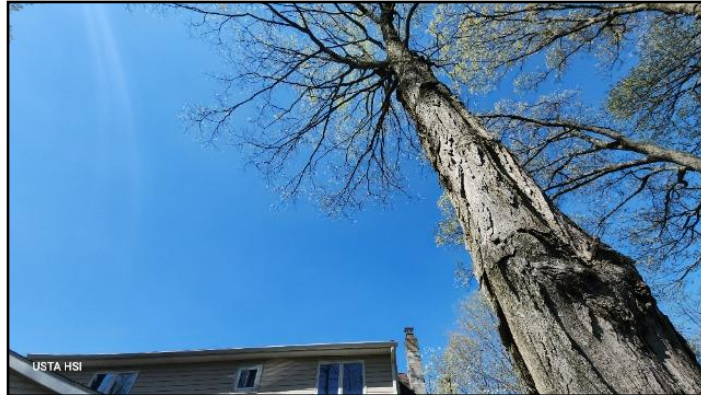
Tree branches were observed overhanging the...
