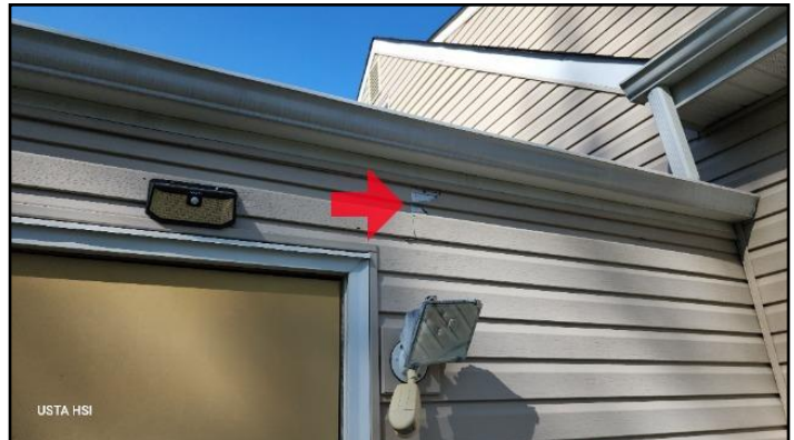
Mechanical damage to the vinyl siding was...
