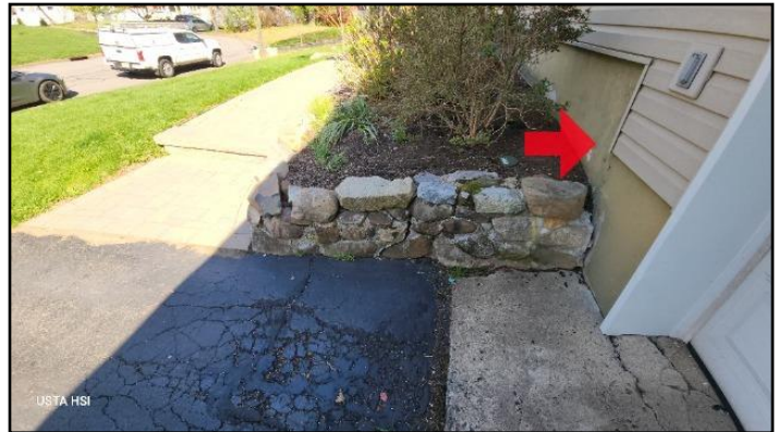
Minor cracks were observed on the exterior...
