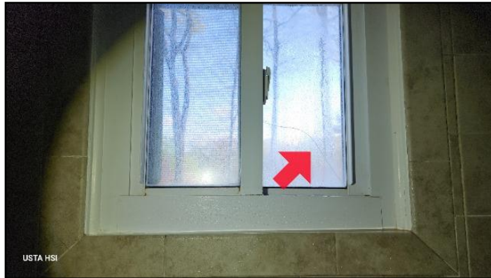
Broken or cracked glass was observed on one...
