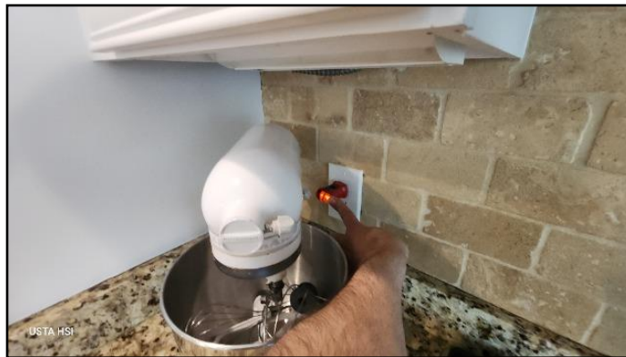
A loose electrical outlet was observed.
