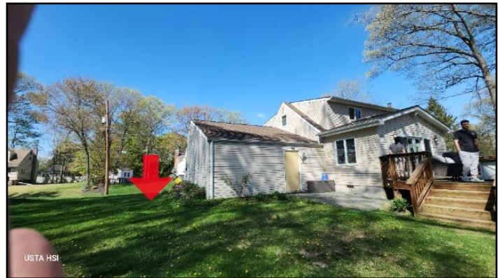
Depressions were observed in the ground...
