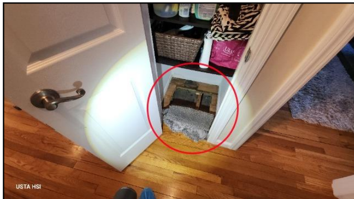
Unfinished floor surfaces were observed.
