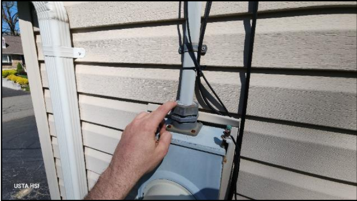
The conduit or cable for the electrical...
