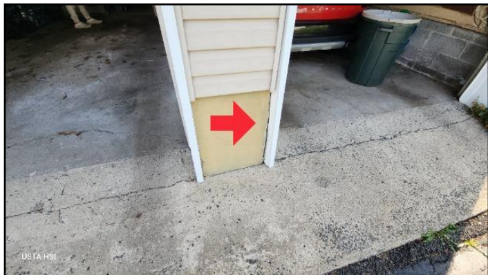
Damage and separation were observed at the ga
