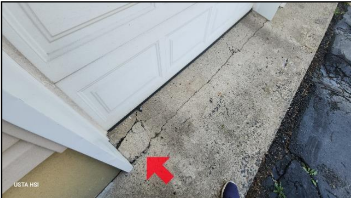
Cracking and deterioration were observed in...
